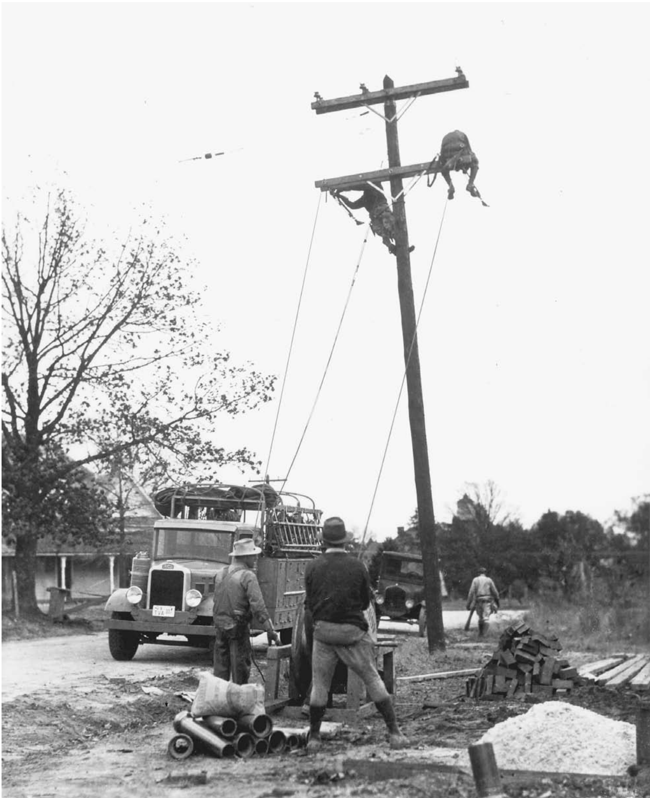
REA workers string transmission line in the Tennessee Valley region during the 1930s. FRANKLIN DELANO ROOSEVELT LIBRARY
