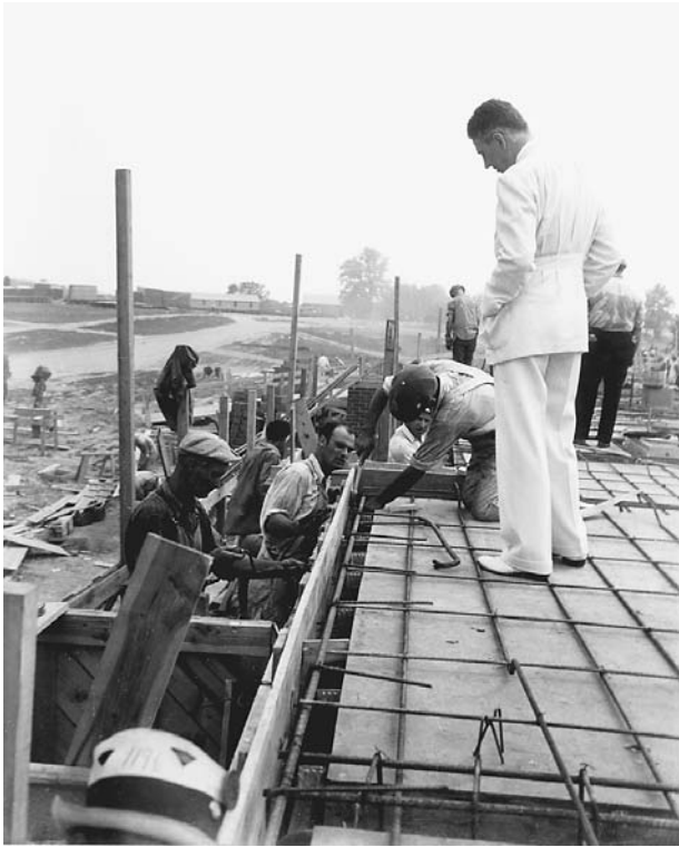
Rexford Tugwell (standing) inspects the foundations of houses under construction at the Greenbelt project in Maryland in 1936. LIBRARY OF CONGRESS, PRINTS & PHOTOGRAPHS DIVISION, FSA/OWI COLLECTION
