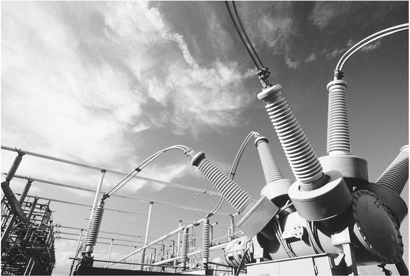
Power transformer station in South Carolina. (Corbis-Bettmann)
